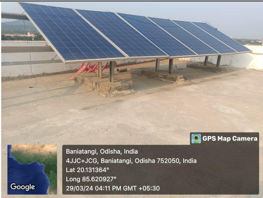
A mini solar power plant has been installed in our campus for production of green and sustainable energy (made by EE & EEE Students)
