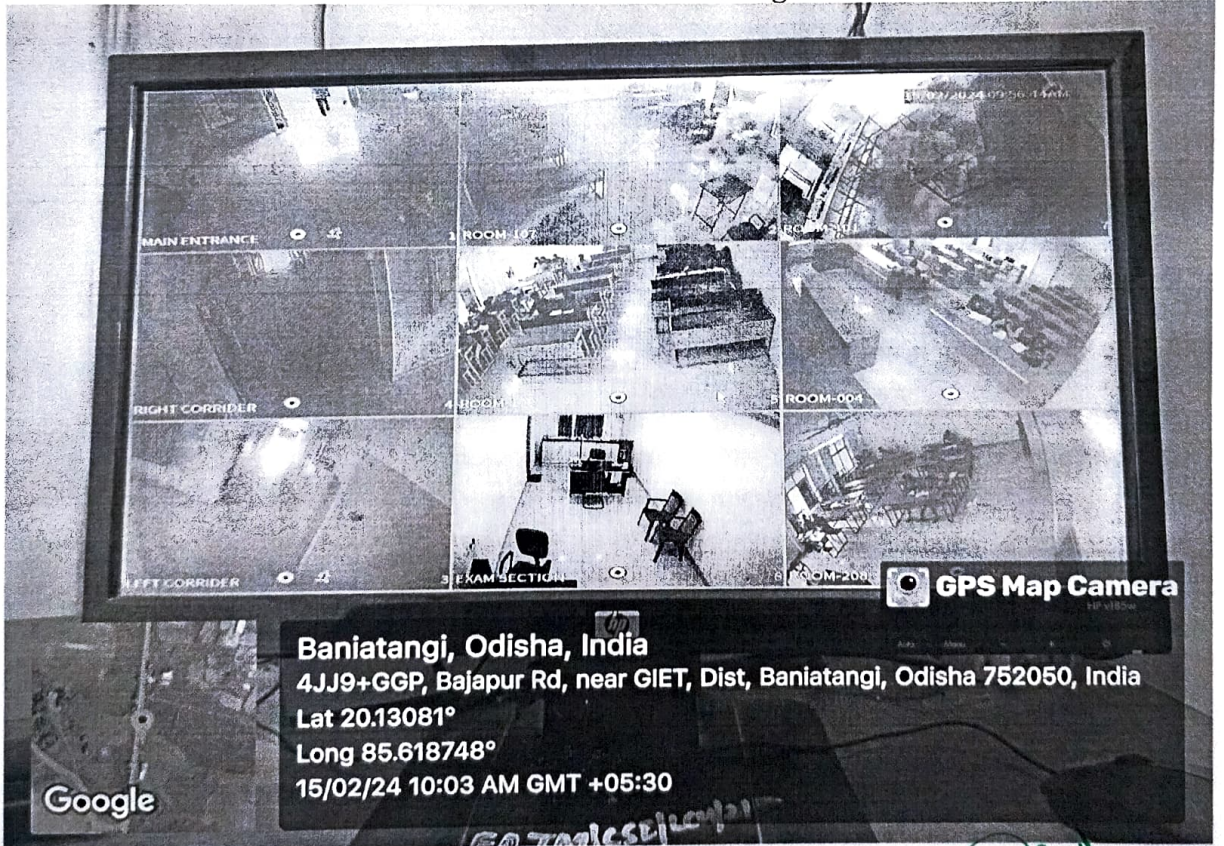
Display of the control room of CCTV cameras of building corridors
